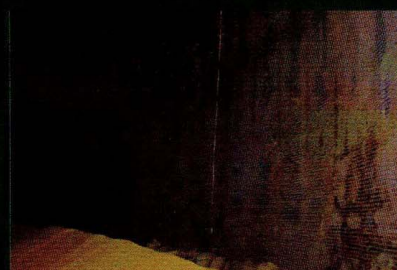
3 years old silo - Heavy corrosion due to constant sweating
